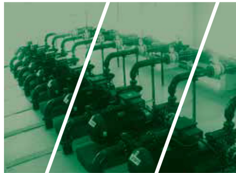
Boosting and Distribution of surface water
