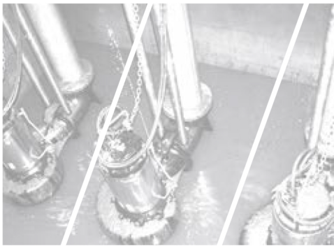
Wastewater Transport and Treatment
